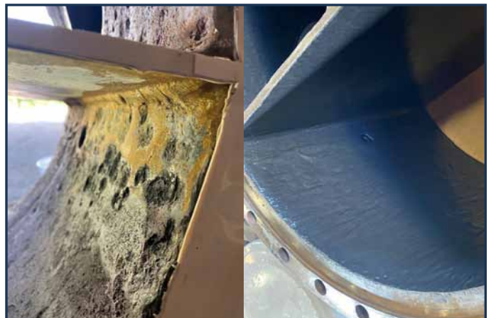
Contrasting images of before and after Curran coating, generalized pitting found across channel and nozzle IDs.
