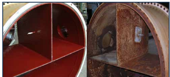
Exchanger cooling water channel, protective coating was used to augment the use of anodes in corrosive cooling water service. Channel coating selection should consider cold wall risk, and exposure to high temperature excursions and steam out.
