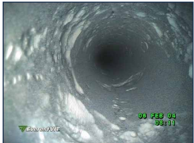
White metal clean ID; corroded exchanger tube in cooling water service
